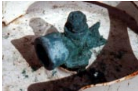
corroded POL valve
