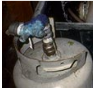
modified valve using galvanized and brass components including a standard brass propane valve (corroded to a blue color) this tank contained ammonia
