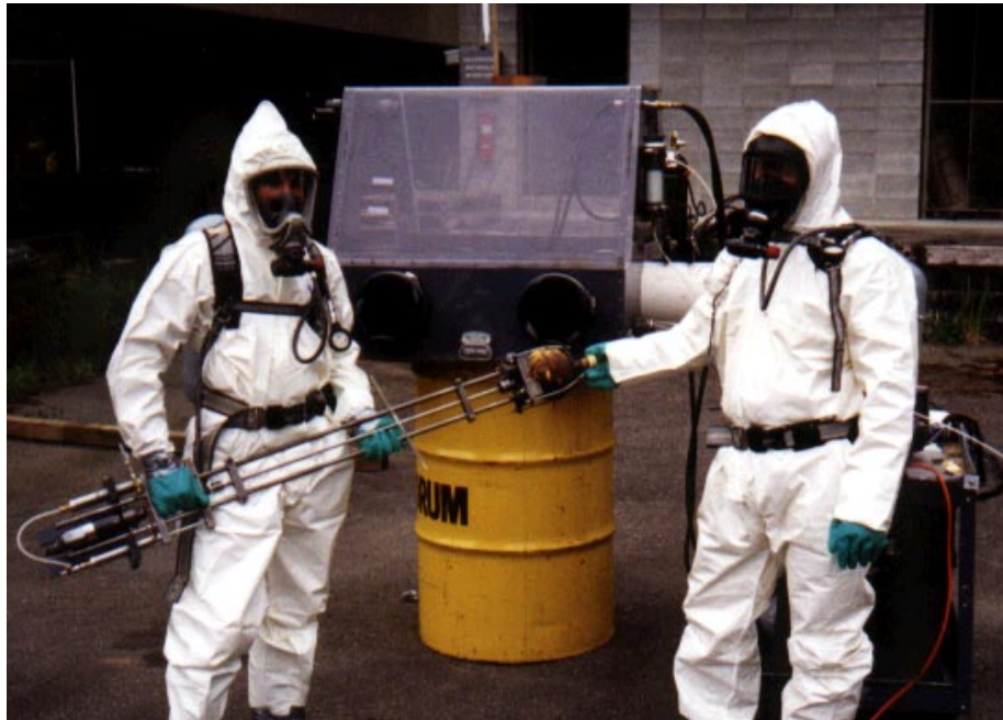
specialized contractor setup with remote drilling unit, scrubber unit and containment hood
